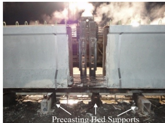
PPCB ends between the bed supports
